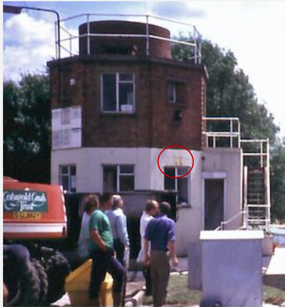
Figure 15: Photo known to be from May 1994 with no lead flashing and evidence of rust staining circled © Stonehouse History Group
