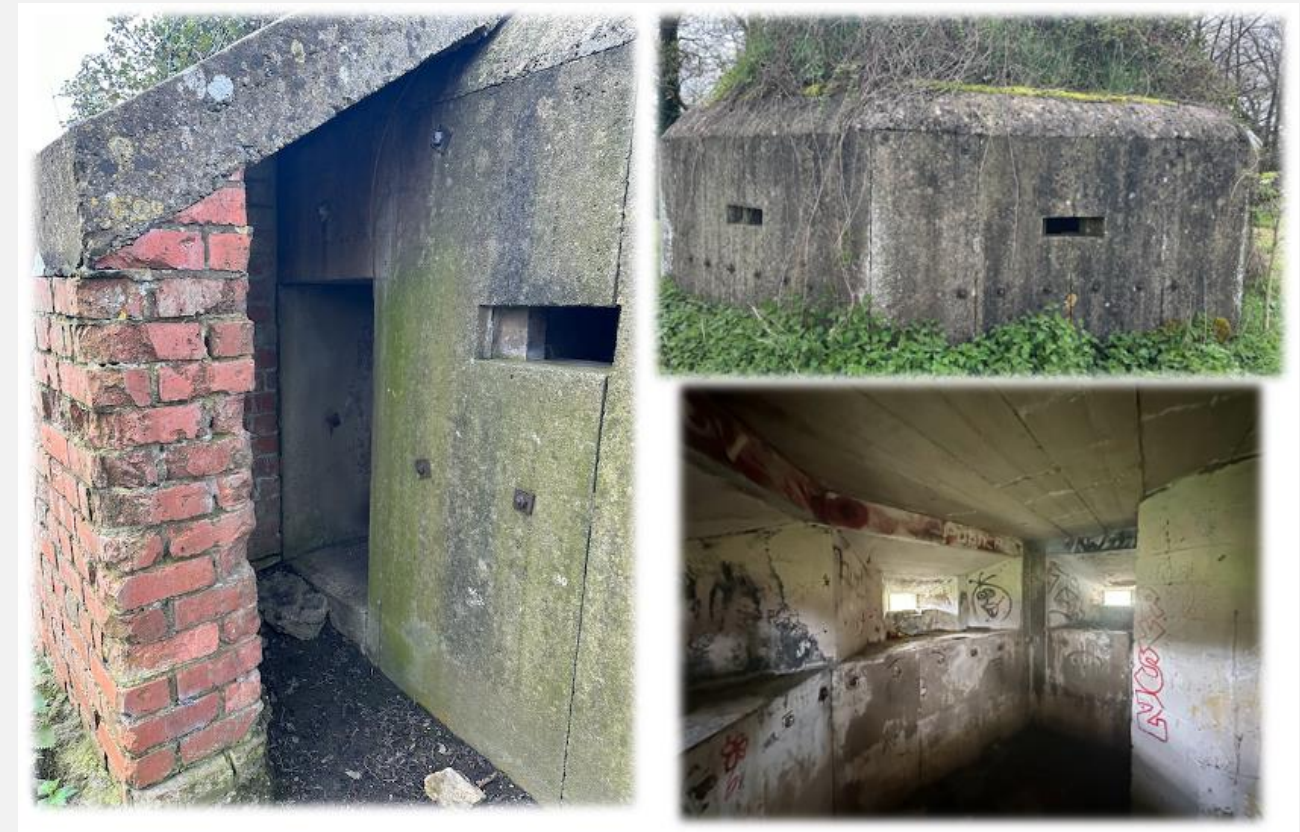
Figure 27: The reinforcements seen at the pillbox south of Bond's Mill which include reinforced entrance porch, iron bolt reinforcement to thicker walls along with a ricochet wall
