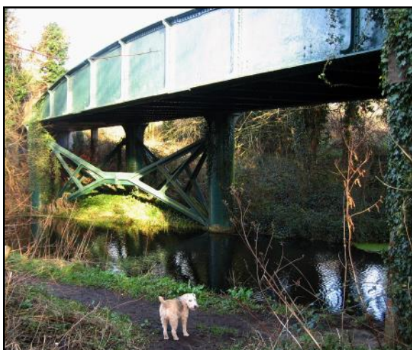
Skew Bridge, 19th January 2007. The cast iron support pillars and their cross ties are clearly visible.
