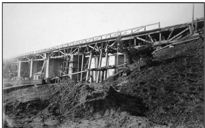
Figure 3. The gradual replacement of the wooden viaduct in the early 1880s, with part of Brunel's structure still visible.
