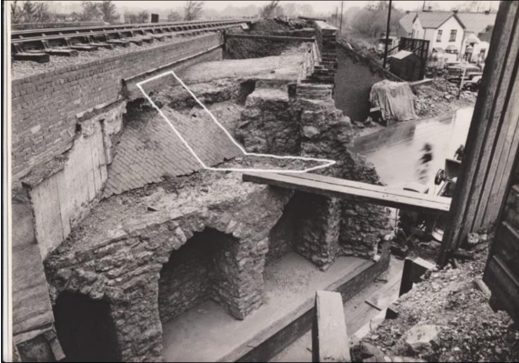
Photo 1: looking west, shows higher skin of brick vaulting resting on the stone arches, stone wall under bridge behind arches, stub of end stone wall
