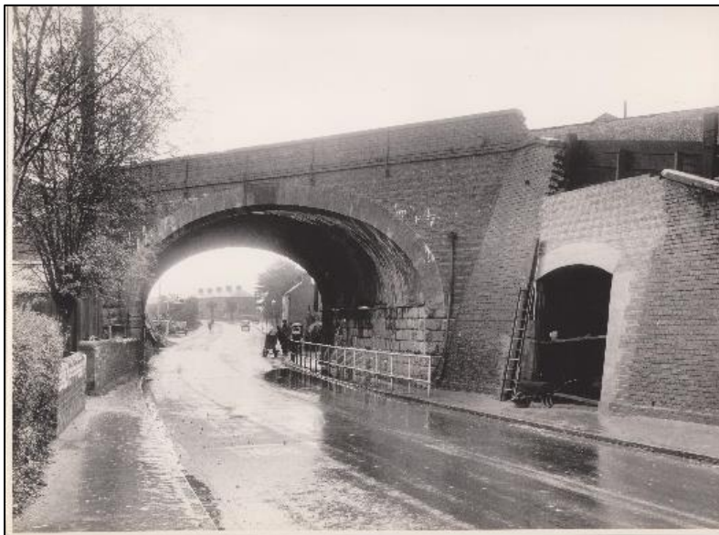
Photo 6: looking north, the bridge arch in 1957, shows stone walling at the base of the bridge arch, supporting the brick vault. The outer face of this stone has since been replaced by brick. The hidden stone arches are about twice as tall as the visible stone wall
