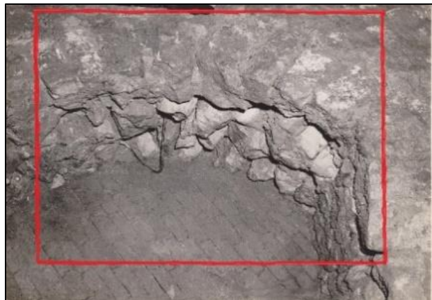
Photo 3: detail of photo 2, area edged red, looking up under stone arch, shows roughly finished surface, and metal tie
